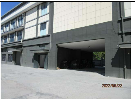
Photo 66) NC 5.5.2 The loading and unloading area was not covered in the factory.
