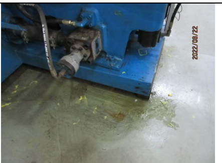
Photo 69) NC 7.4.5 One vulcanization machine leaking oil
